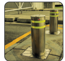
Vehicle Barriers & Bollards
